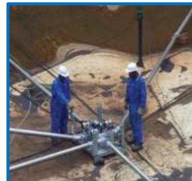
ARRAY 8 - 16 SPRAY NOZZLES
