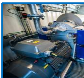
ATC 3-PHASED DECANTER
