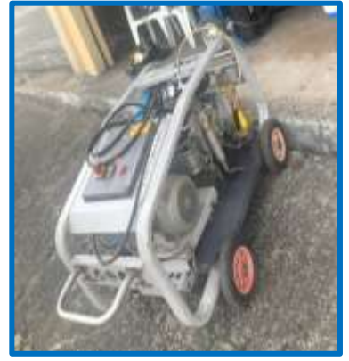
Breathing Air Generator
