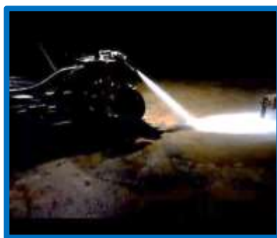
REMOTE-OPERATED JETS IN TANK
