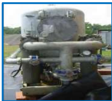
ATC SUCTION MODULE-1
