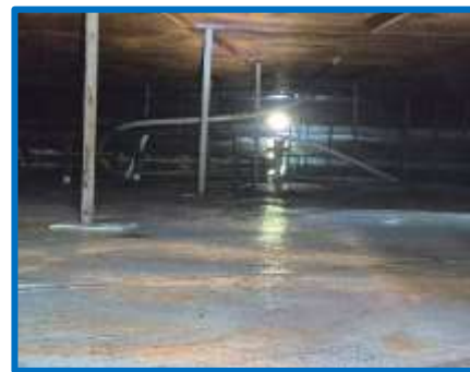
ATC NME WELL-CLEANED TANK
