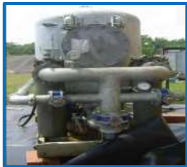
ATC SUCTION MODULE-1
